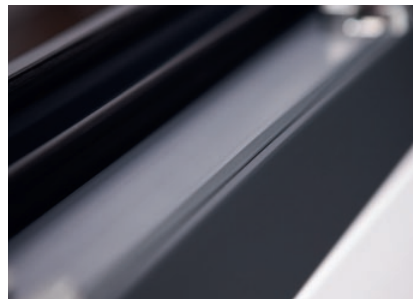
Infilled bottom groove
